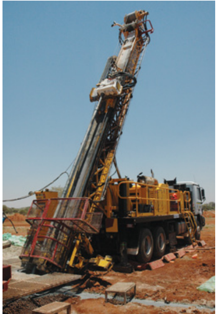
Although the blitz of drilling to upgrade the Andy Well resource is now over, three drill rigs remain on-site. The diamond rig is testing the southern extensions of the Wilber Lode resource here
